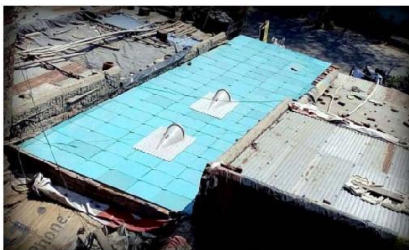
Figure 11: ModRoof installation in Ahmedabad by Mahila Housing SEWA Trust (Mahila Housing SEWA Trust, 2016)
