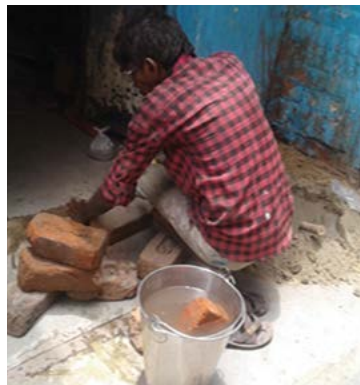
Construction of brick embankments "Palis" by using bricks and cement at a house of slum dweller.
