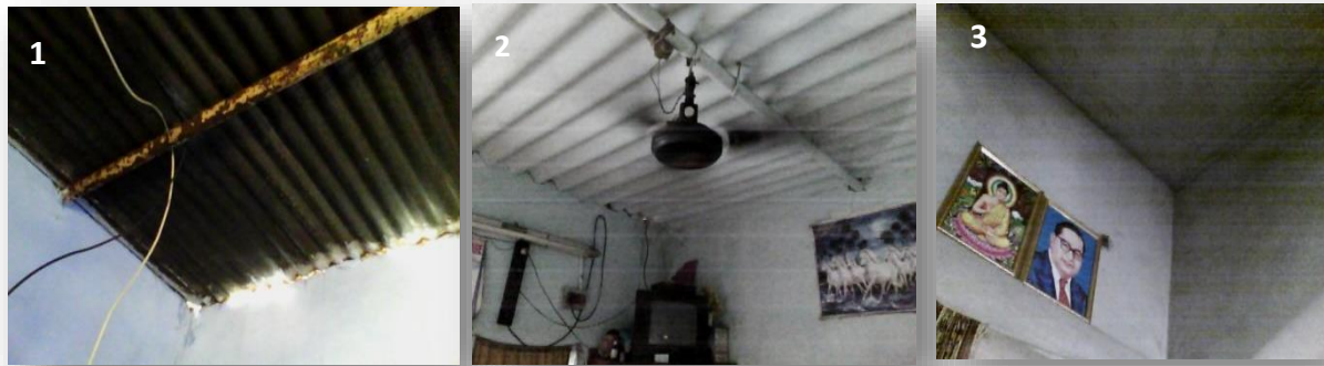
Figure 3: Control roof types - Right to Left 1.Tin Roof, 2.Asbestos Sheet and 3.RCC Concrete roof
