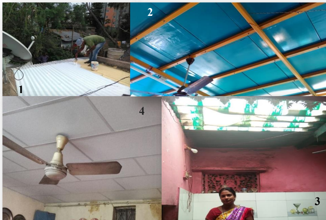
Figure 2 : Four Intervention roof types: Clockwise 1.Solar reflective white paint, 2. Modular Roof, 3.Air-lite Ventilation and 4.Thermocol Ceiling
